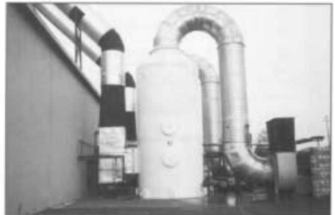
MCBS on the Press Exhaust for Formaldehyde scrubbing.
