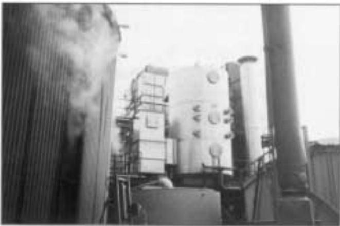
MCBS on the Dryer Exhaust for particulate and cooling.
