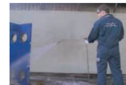
9. Frame reconditioning. If required, inspection and power washing of frame assembly and covers. Sandblasting and painting are optional.
